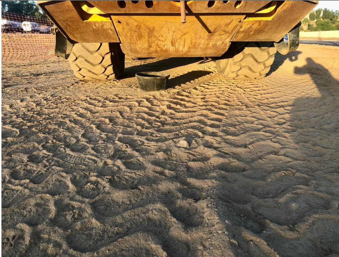
Photo 11 – Secondary containment under some equipment – note the small size. The area could use some dust control.
