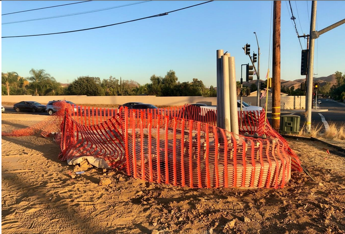
Photo 9 – At TSP #302E the foundation has been poured and some fencing installed. Photo facing south
