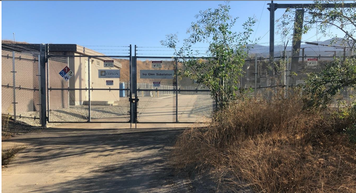
Photo 4 – Entrance to the Ivy Glen Substation. Photo facing southwest
