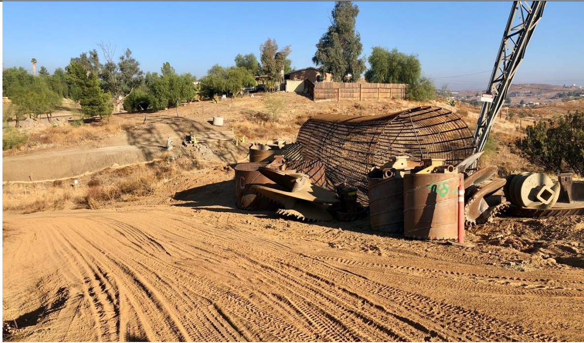
Photo 10 – Access road to tower site 144 with staged drill bits and rebar cage. Photo facing north
