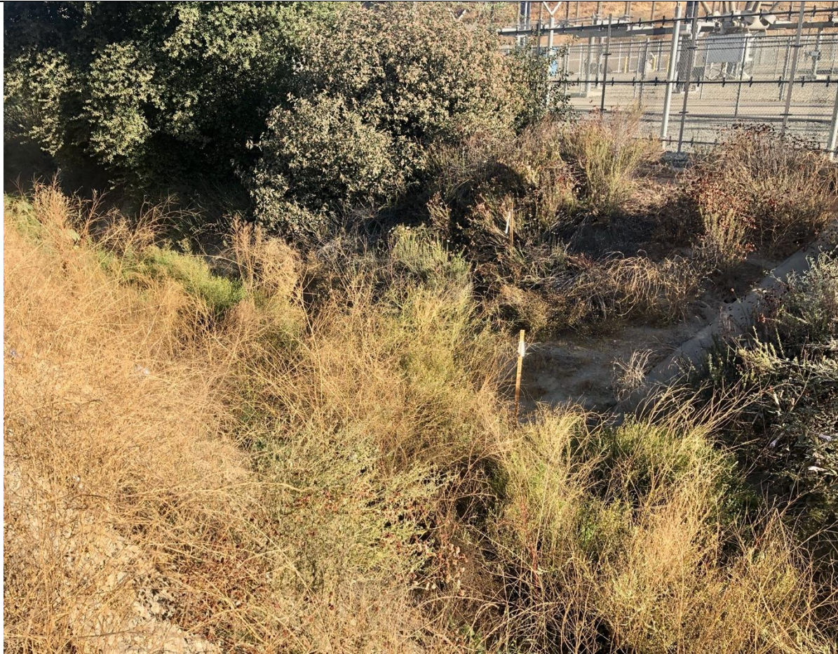
Photo 5 – Pole locations within the drainage just outside of the Ivy Glen Substation. Photo facing south
