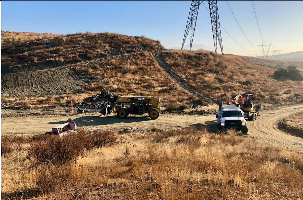
Photo 6 – Filter fabric is being installed at this location along the access road. Photo facing east
